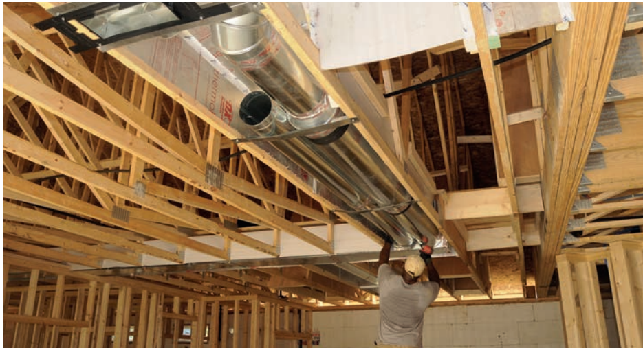
Afbeelding 40: Ductwork. (Bron: Crowl Marketing + creative courtesy Pro Builder Media https://www.probuilder.com/ )
